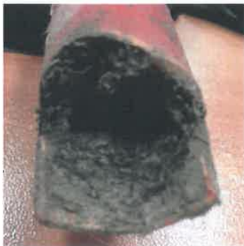
Extreme example of pipes being impeded by excessive
